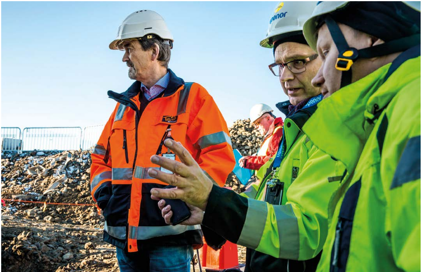
Installation of Uponor's Weholite® at the new sewage treatment plant in Borås, Sweden, where secure pipes and fittings are vital.
